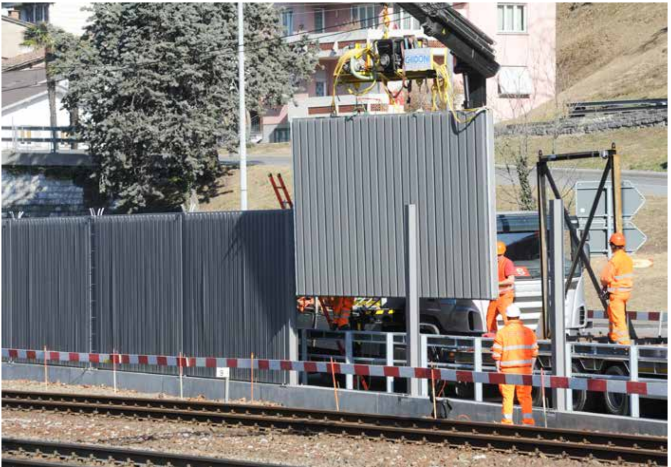
Workers during the installation of noise barriers on the railway. © istock / fotoember
